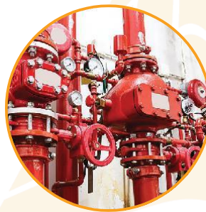
Fire protection stations
